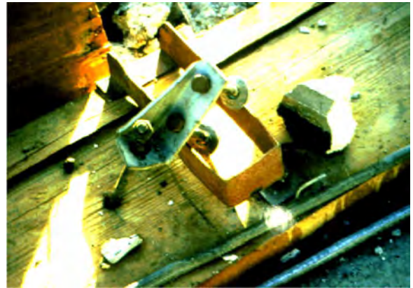
Figure E-38 Tilt-up construction anchorage failure.
