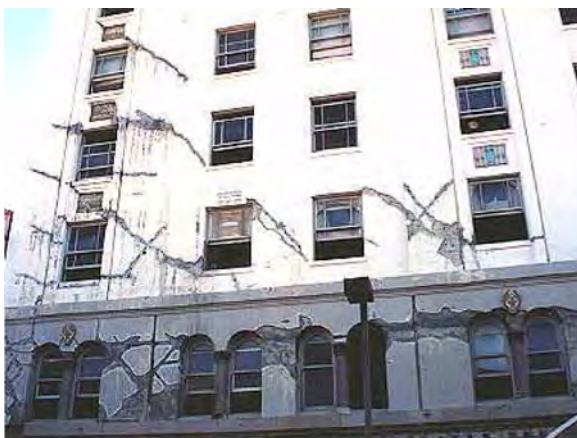
Figure E-32 Shear-wall damage, 1989 Loma Prieta earthquake.
