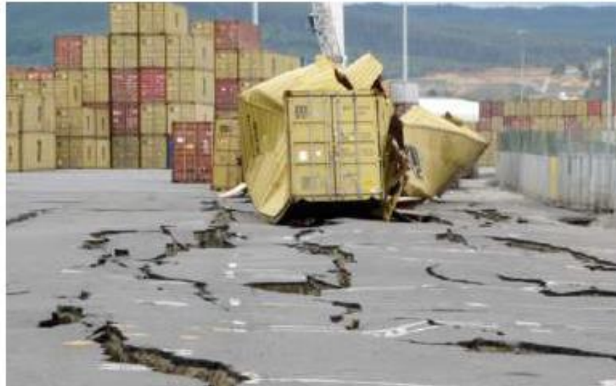
Figure 1-2. Examples of infrastructure damage at a port facility due to liquefaction (from Wang et al. 2013)
